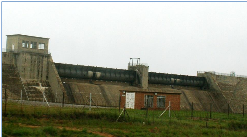
Fig 5 – Position of the artificial ledges being used on Westoe Dam. Both the left and right hand sides of the release gates are used where a flat surface is available on the metal wall. The white-wash is extensive, indicating the ledges have been used for a number of years. There is an additional roosting site on the left below the observation room (CLH).
